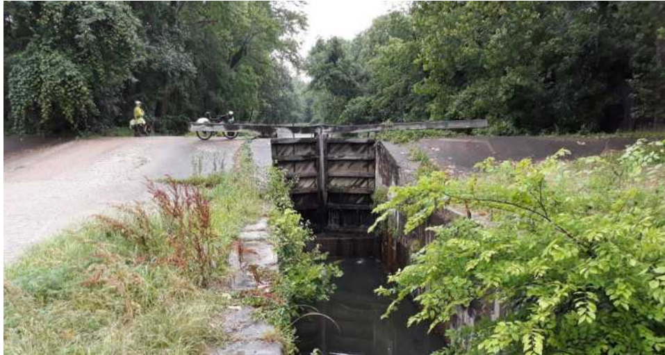
Another view of one of the canal control gates
